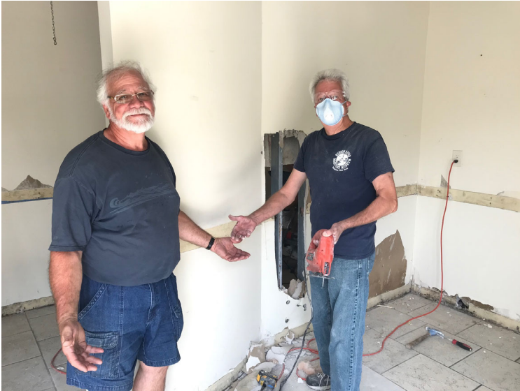
Museum volunteers working on the demolition of the current Wooden Boat School bathrooms.
